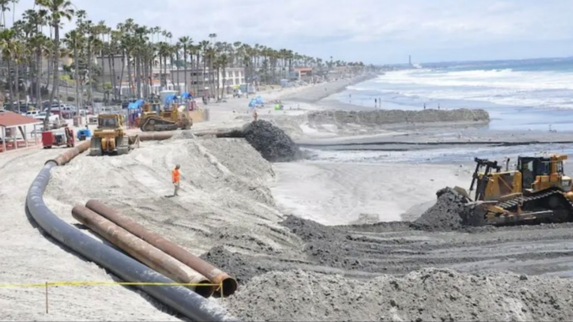
The U.S. Army Corps of Engineers conducts a yearly dredging of the Oceanside Harbor inlet. Photo courtesy of USACE
